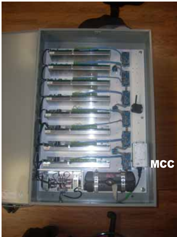
Figure 1-14: Installed iDAC panel and MCC assembly
